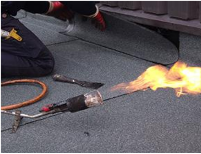
Gas torch unsupervised and abutment to cladding
